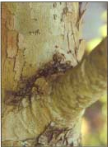
Fig. 7b. Example of strong branch union without embedded or included bark. Note the dark tissue on the trunk just above the branch crotch. This is the branch bark ridge. Its presence above the branch indicates there is no included bark.
